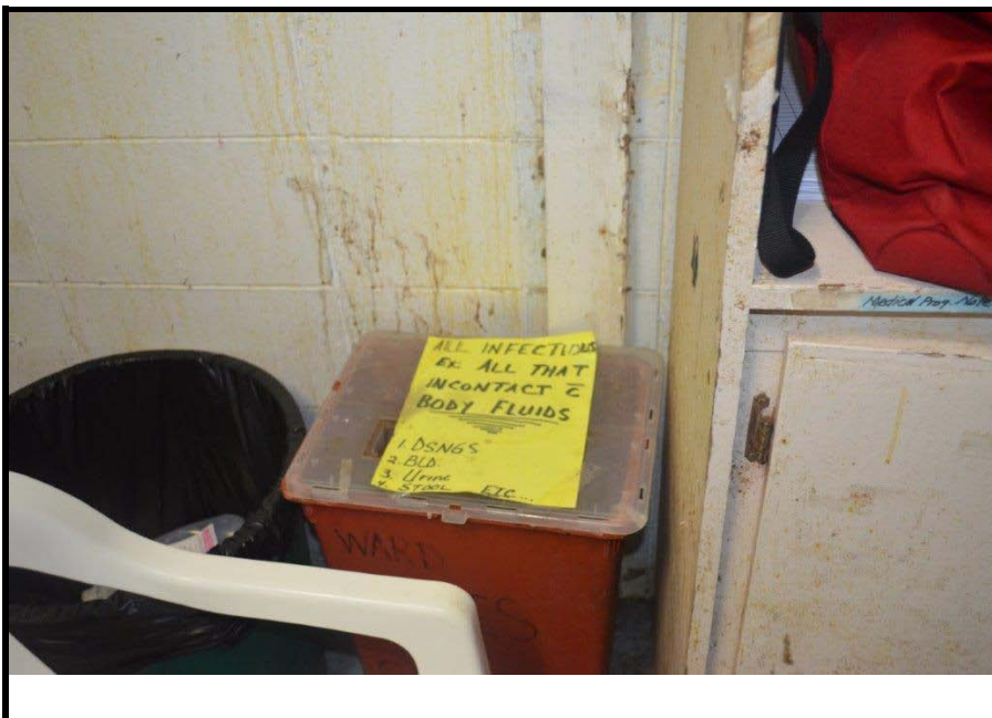
Photo 12: Example of healthcare waste disposal at Kosrae Hospital, signage is limited however where it is present in is handwritten. Dedicated red containers used in some instances. (taken 8/04/2014 by Natalie Stella ref:DSC0413)
