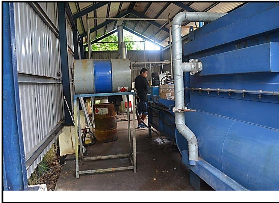
Photo 7: Second incinerator visible in photo no outlet for stack exhaust (taken 4/04/2014 by Natalie Stella ref:DSC0139)
