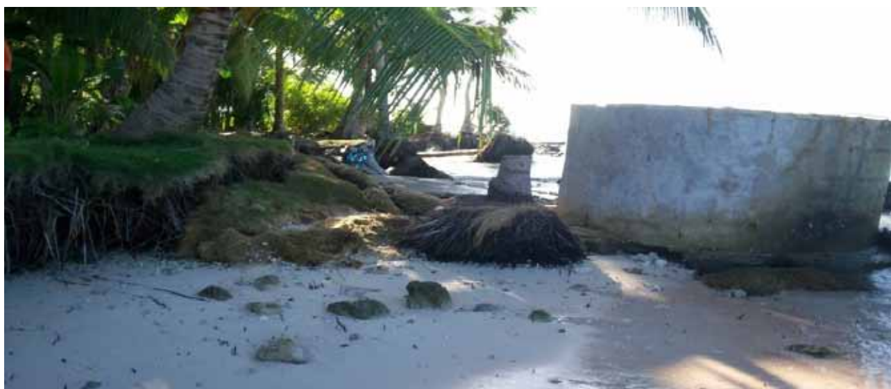
Coastal erosion on Polap atoll Chuuk by Henry Susaia
