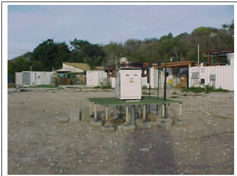
ARM Project site and installed monitoring equipment.
