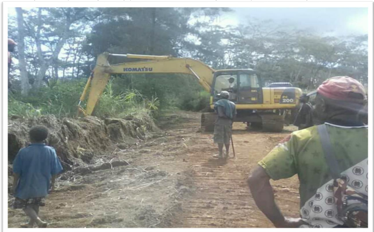
Image 7: Image 4: Civil Works (Clearing and Grubbing) resumed yesterday (Tuesday, December 11, 2018) at Pubi-Paiyama area after the consensus reached between locals and HRMG during the discussion held on Monday, December 10, 2018. Locals have now agreed to allow the work to proceed. Pic. Courtesy of Site Engineer-PWL.
