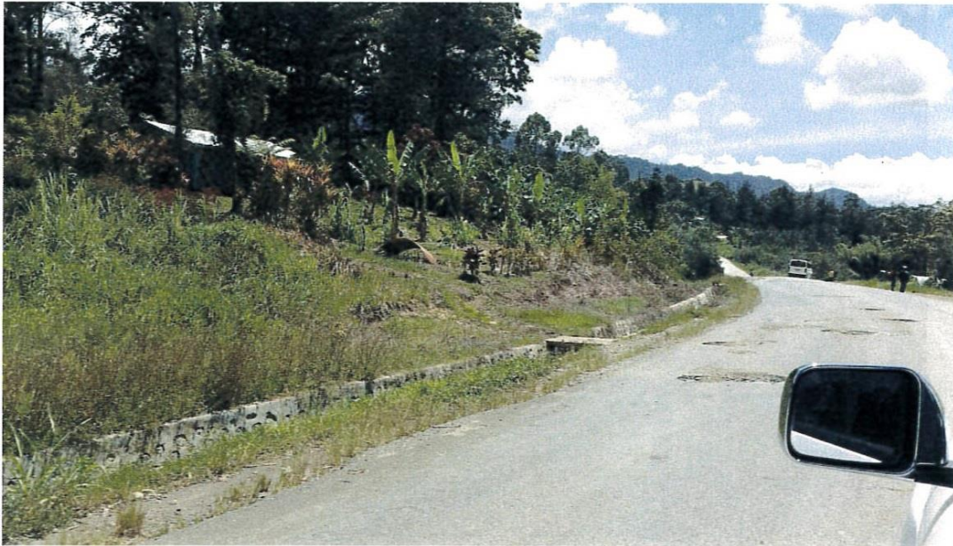
Photo 15 showing a section typical to zones 2 - 5, with frequent potholes
