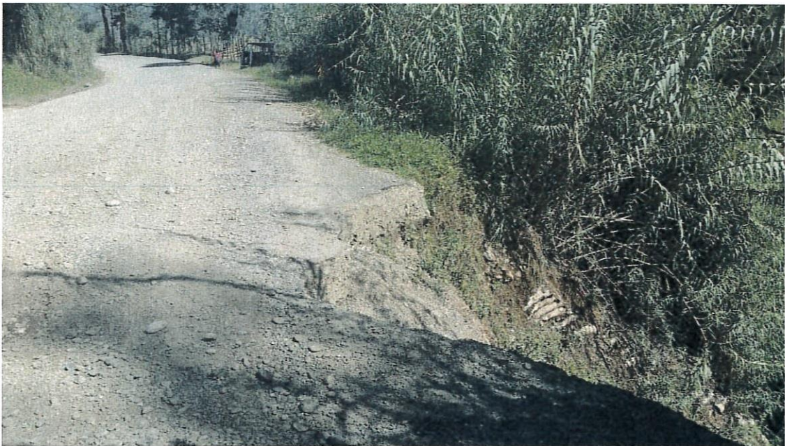
Photo 14 showing severely degraded pavement and effects of regressive erosion, in Zone 3
