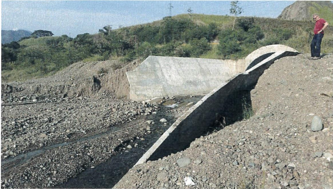
Photo 17 showing the damaged wing outlet to the culvert near Leron Bridge. This culvert had been recently constructed with support from TSSP. Several meters of the wing on the far side have been washed away by recent floods
