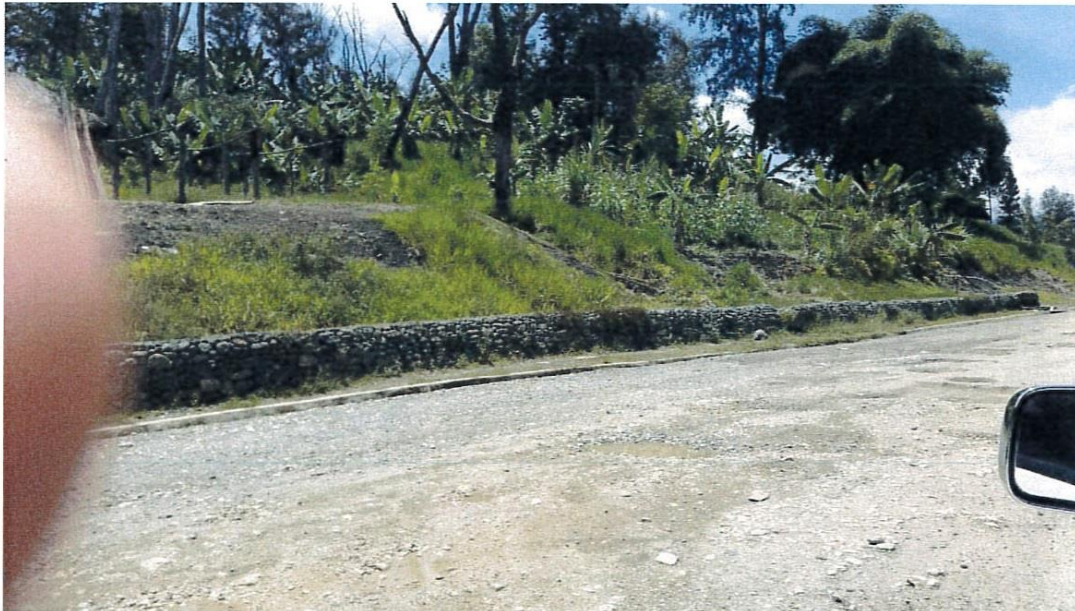
Photo 16 showing a severely degraded section, with deformation and potholes (Zone 3)
