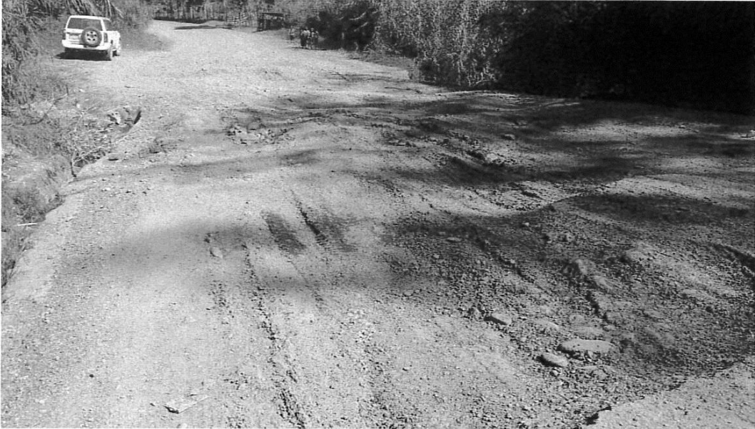
Photo 11 showing an example of severely degraded pavement, in Zone 3
