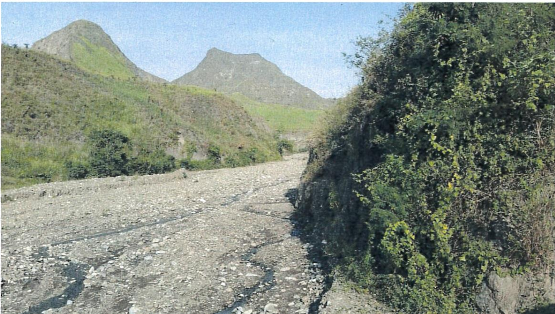
Photo 18 this is the stream that caused the damage to the culvert in the previous photo. The catchment area is clearly visible
