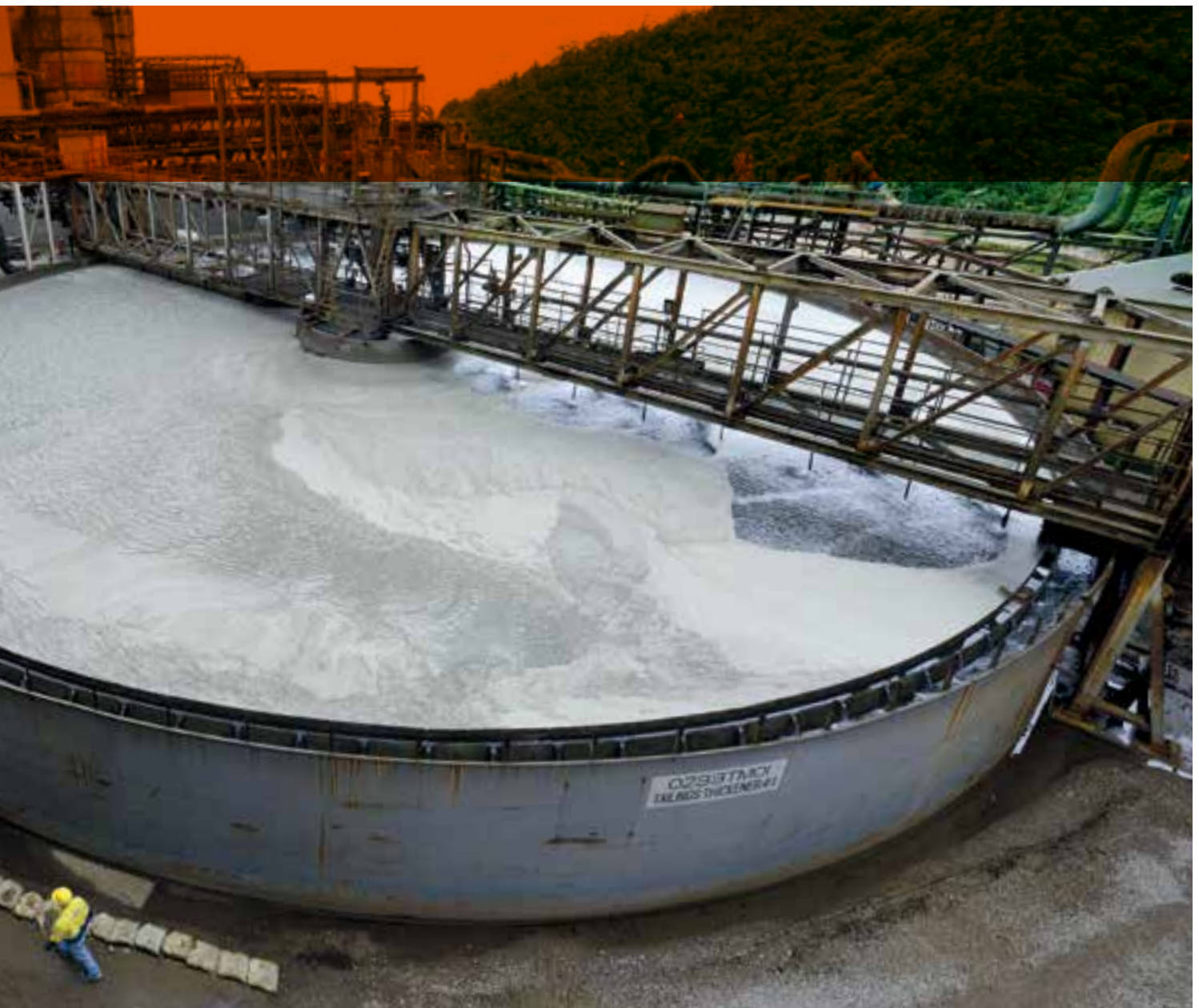
| ABOVE: Processing plant tailings thickener.
