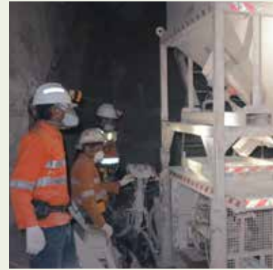
Employees at Toguraci operating the grouting pump to consolidate material above the sill pillars prior to stoping.
