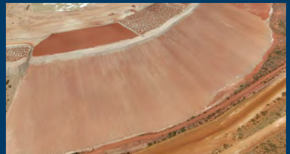
Almost 60 hectares has been rehabilitated at our Telfer mine site and work is continuing.
