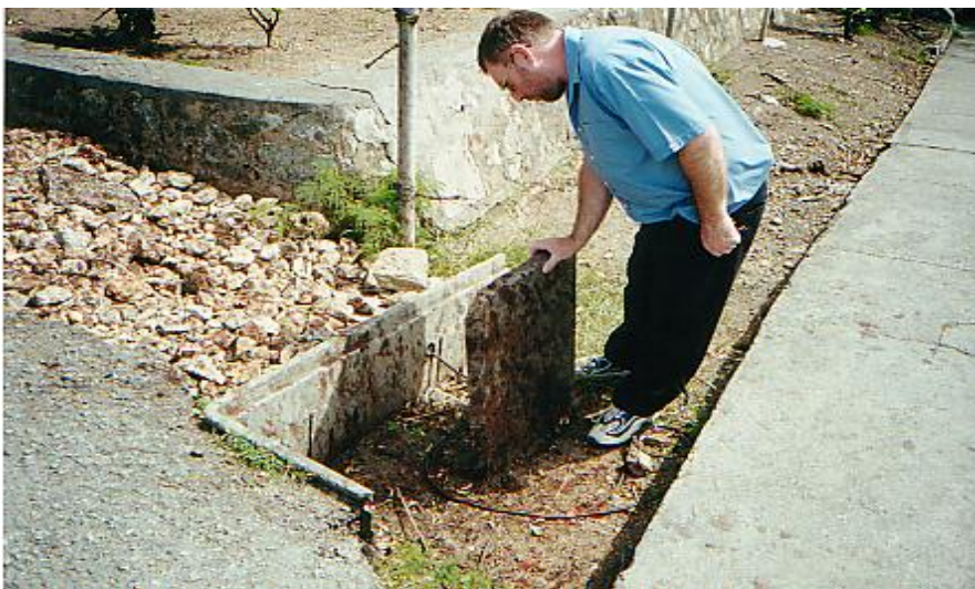
Photo 22: Flood- damaged Telikom Pit
