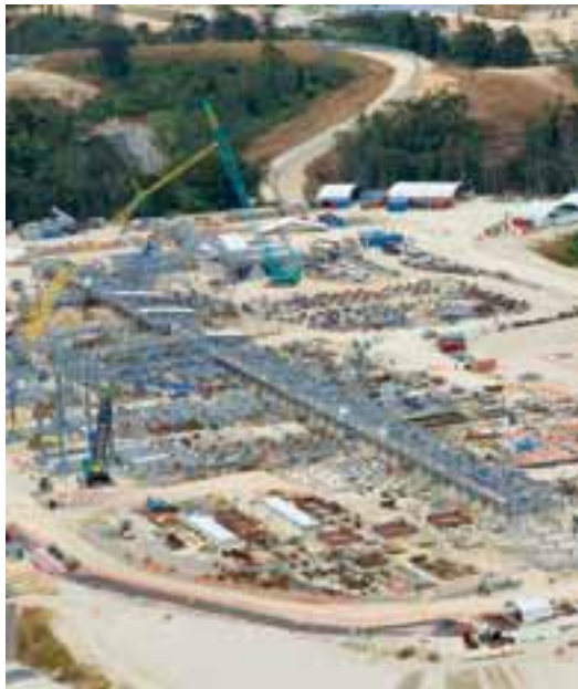
Initial geothermal development was carried out for mining purposes
