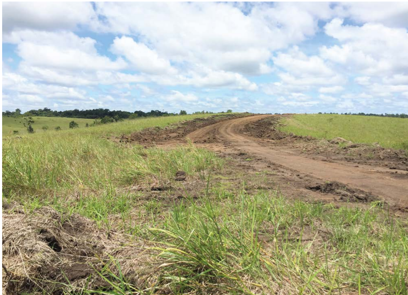
First stage of an alleged new road line project, also serving as a forest access road; Turubu area, East Sepik Province. ©Global Witness 2018
