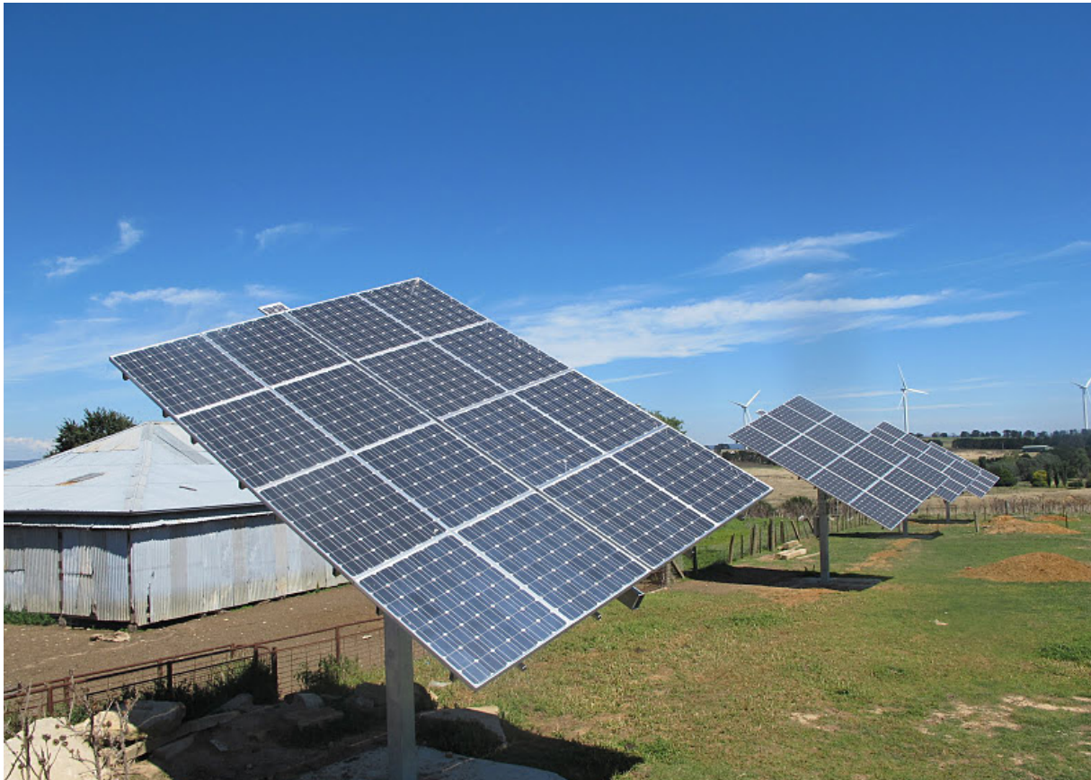
Solar panels in the Australian bush
