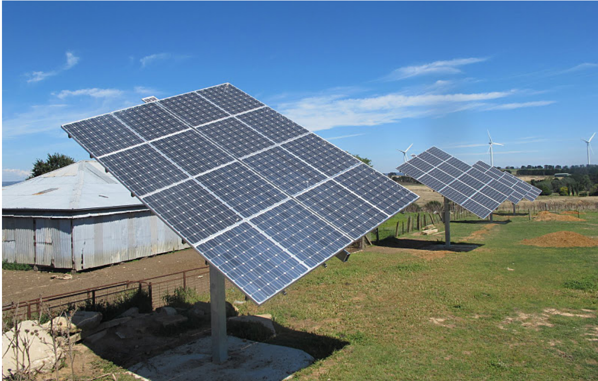
Solar panels in the Australian Bush
