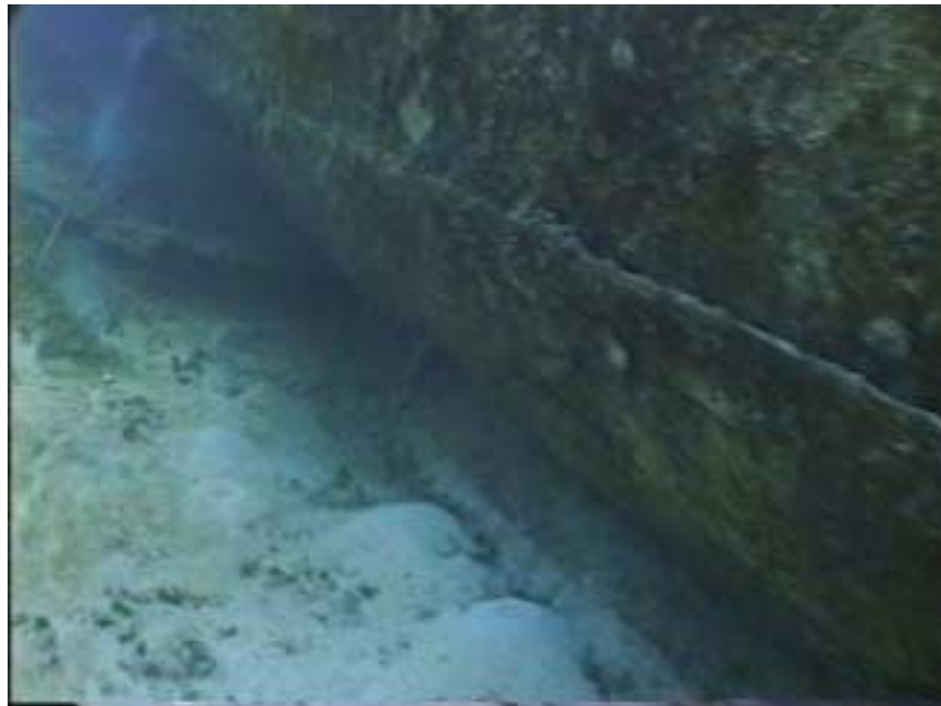
Photo KS4-7 Steel sheeting added to below the waterline. Note section fallen away at top left of photo which is next to the engine room.
