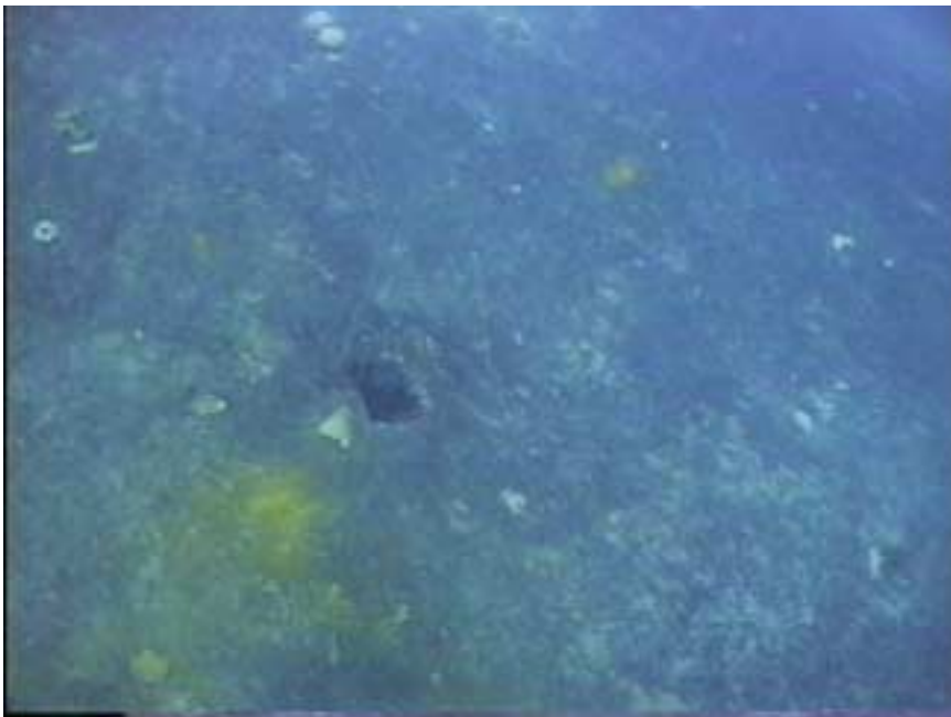
Photo WT12-17. Small hole in stern on starboard side, probably from Naval artillery shell.
