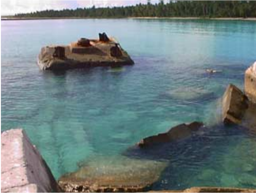
Photo WT6-2. Deep end of Main Service Dock, heavily damaged by bombing and time, with crane base exposed on original end of dock.
