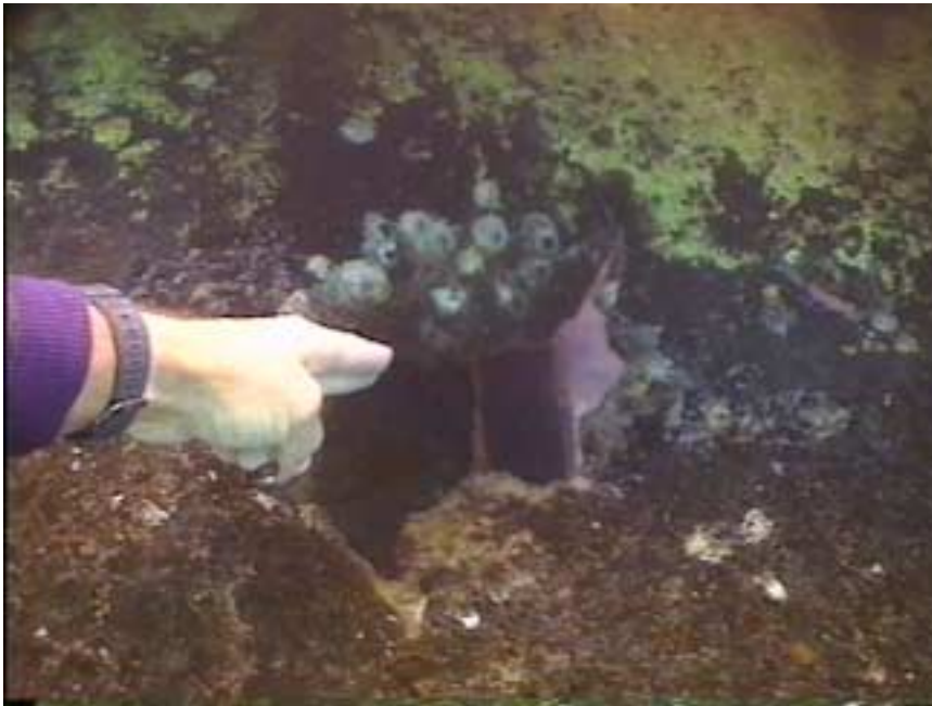
Photo WT13-7. Hole likely from artillery shell, but also possible damage from a near bomb explosion.
