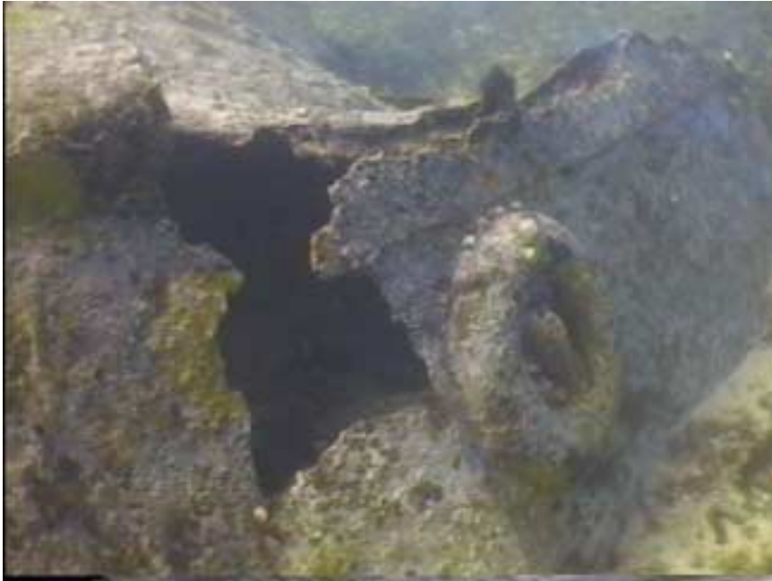
Photo WT9-2. Bow of steel vessel with chain tube opening. Note rust mark at false waterline, indicating vessel rotted for along time before being demolished.
