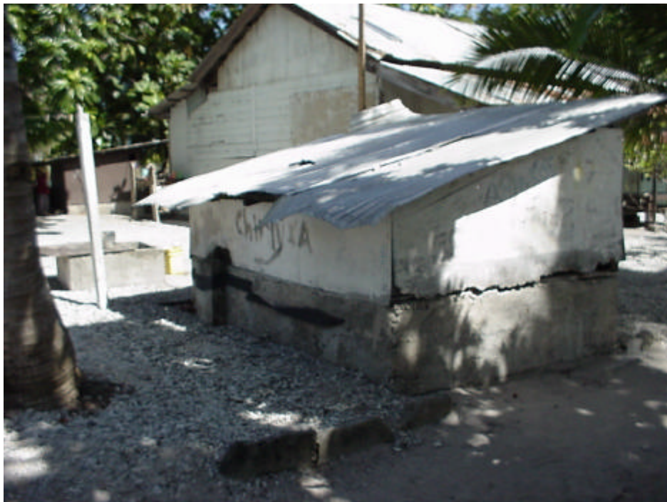
Photo 3 Water Catchment at Jaluit Company Trade Station
