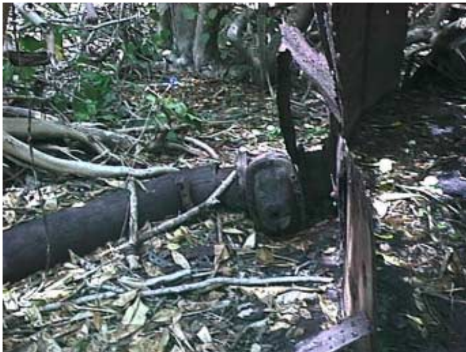
Figure 6. Pipeline Running Outside of Tank 3.
