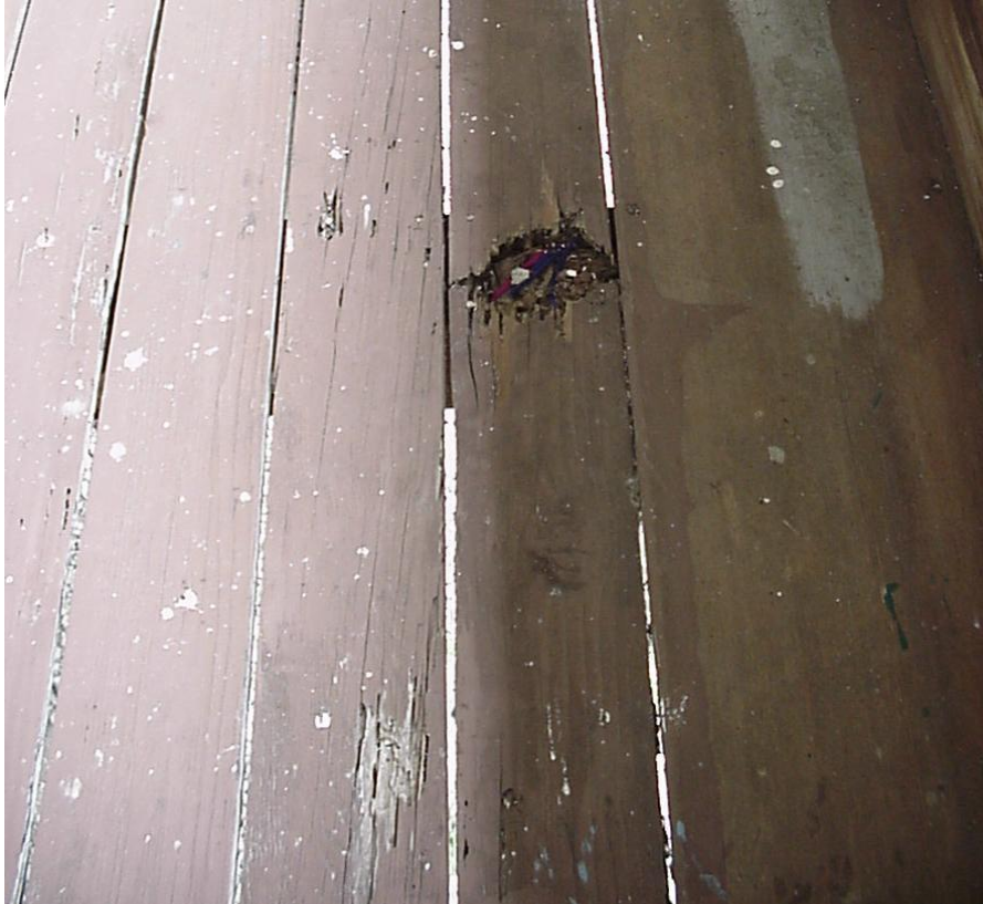
Photo 14: Termite damage on reconstructed portion of east veranda.
