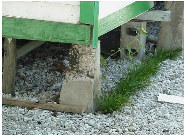
Photo 58: Close up of deteriorating pillar from Godfrey Capelle house.
