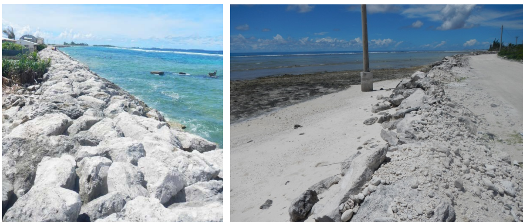
Figure 1.6 Left picture: well-constructed revetment. Right-picture: poorly constructed revetment.
