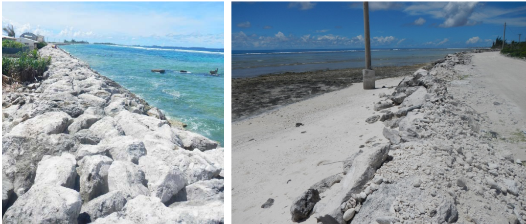
Figure 7.17 Left picture: well-constructed revetment. Right-picture: poorly constructed revetment.
