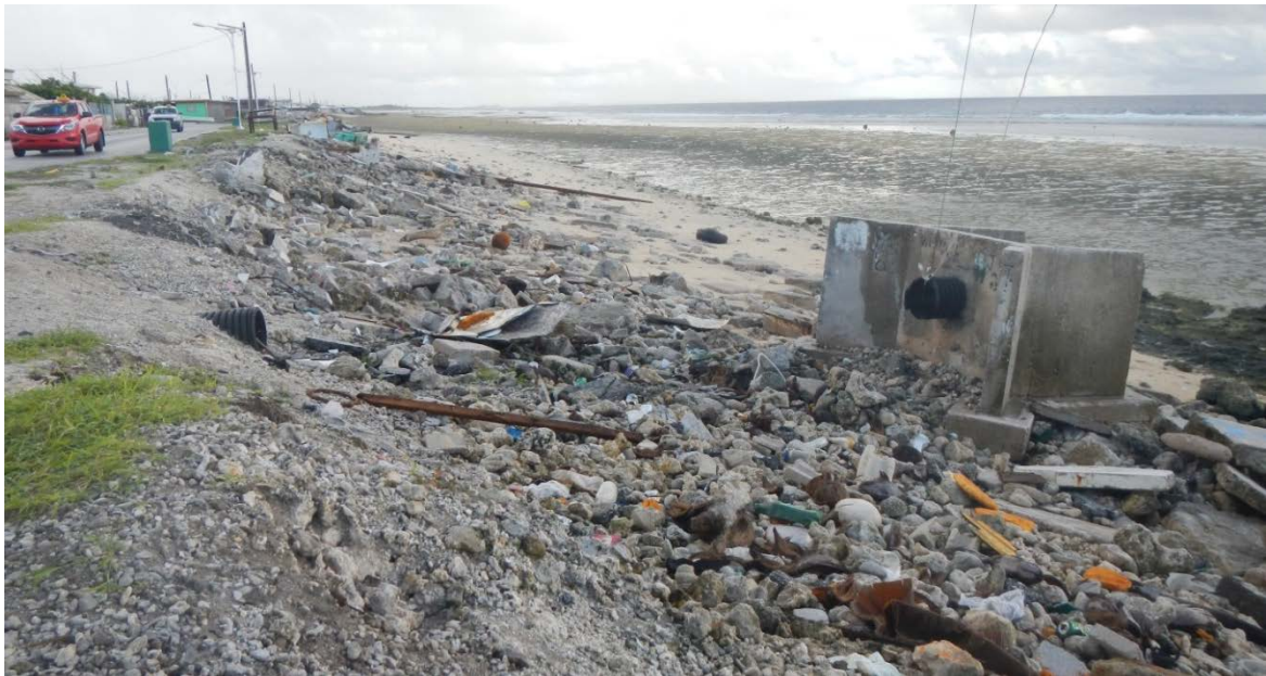
Figure 7.20 Coastal erosion at the ocean side of Ebeye.
