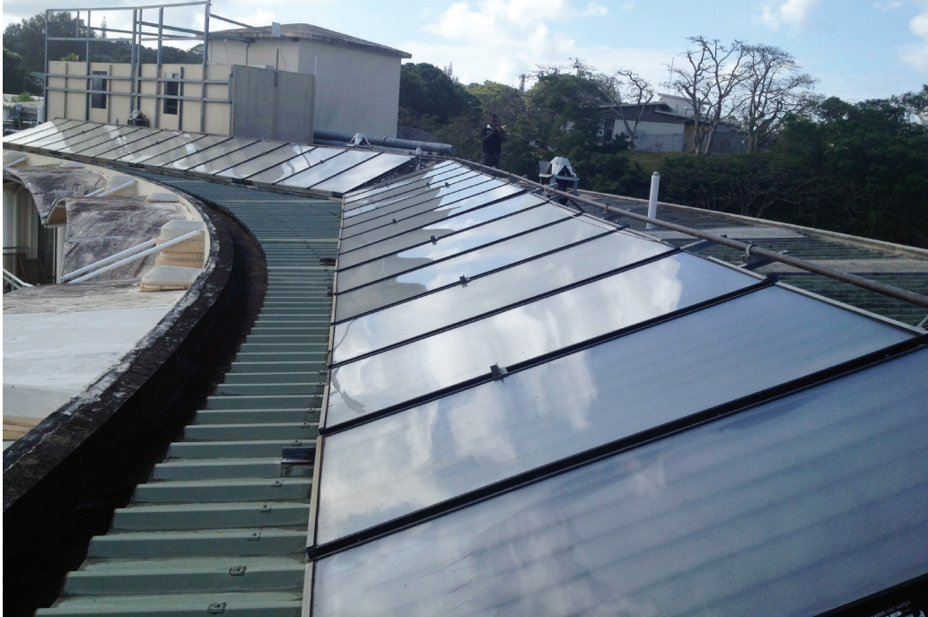
Solar Water Heaters, Grand Hotel Port Vila Photo: H. Wade
