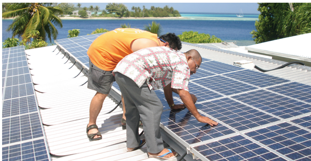
Solar PV for Jica Freezers
