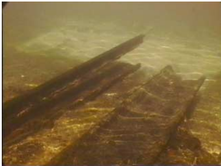
Photo MS7-5 Marine Railway section broken off in the tidal zone.
