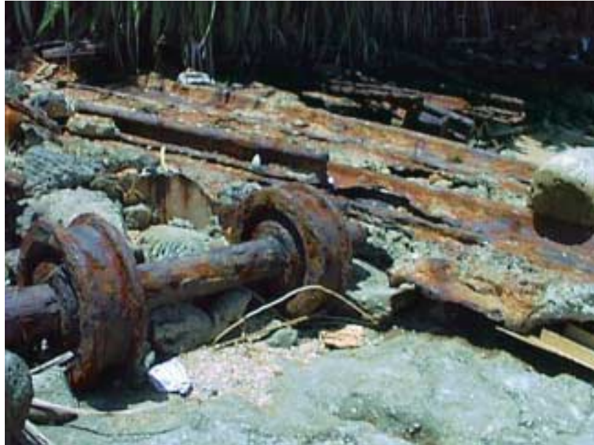
Photo MS7-2 Northern section of Marine Railway at tidal zone during low tide. The wheels are for original carriage to support hauled-out small craft.
