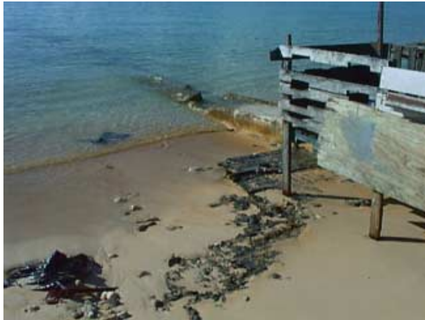
Photo MS8-2 North side of Seaplane Ramp with remains of Marston Matting still embedded in the ground. A pigpen has been secured to the concrete section.
