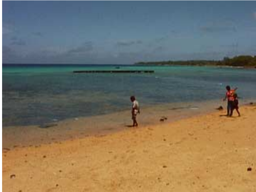
Photo MS6-2 A broken section of Rita US Dock lagoon-side of the shore-side anchoring point. The "Dead-man" on the end of the Japanese Wharf is visible farther behind it, and also the Majuro Site 3 "Parking Lot" directly in line with a compass point (260 degrees) to the post on the shallow coral area near
