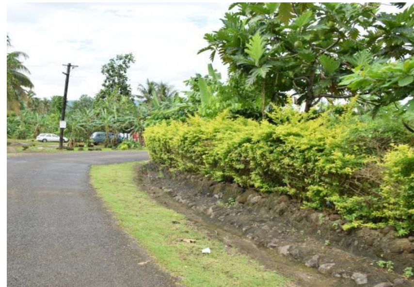
Plate 2: New Subdivision areas – improved table drains
