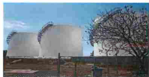
Figure 16: Three new Petroleum Storage Tanks at Apia Wharf
