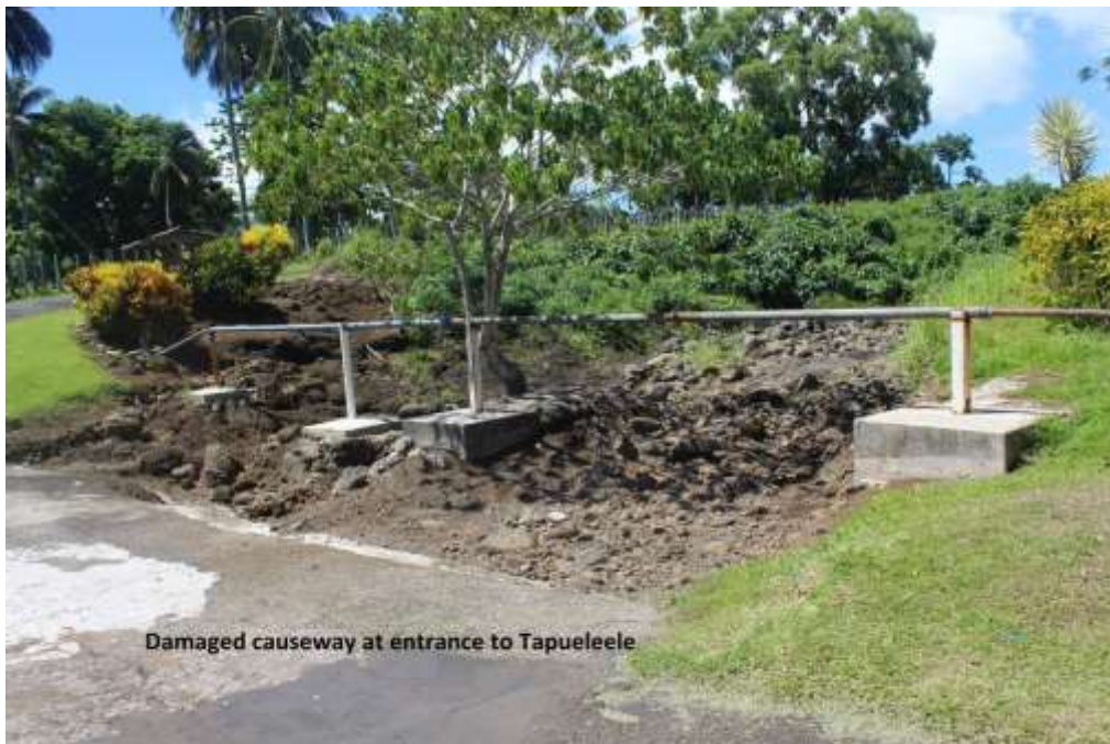
Damaged causeway at entrance to Tapueleele
