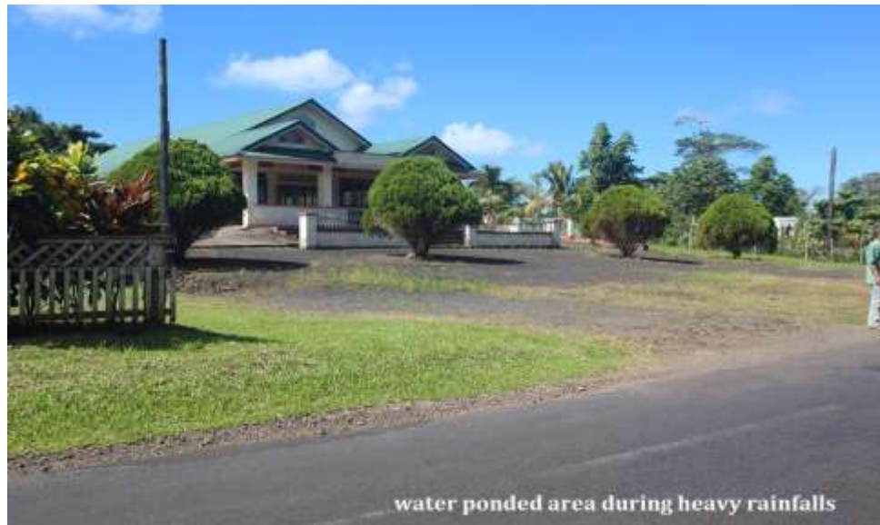
poorly upgraded Tanumalala Access Road
