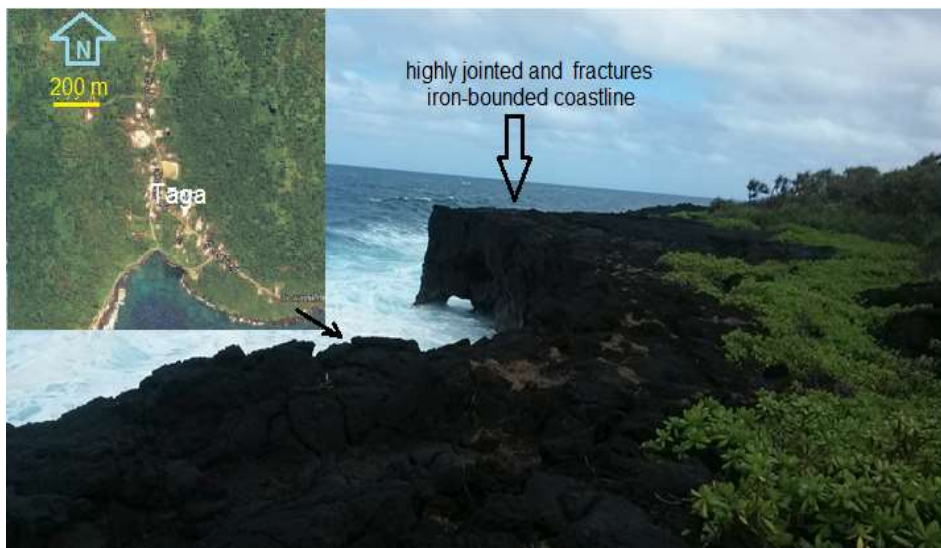
Figure 2 Highly jointed and fractured iron-bounded coastline of Taga. Index image of Taga village shows the actual part of the coast that is vulnerable to collapse Photo credit: Aleni Fepuleai, 2017
