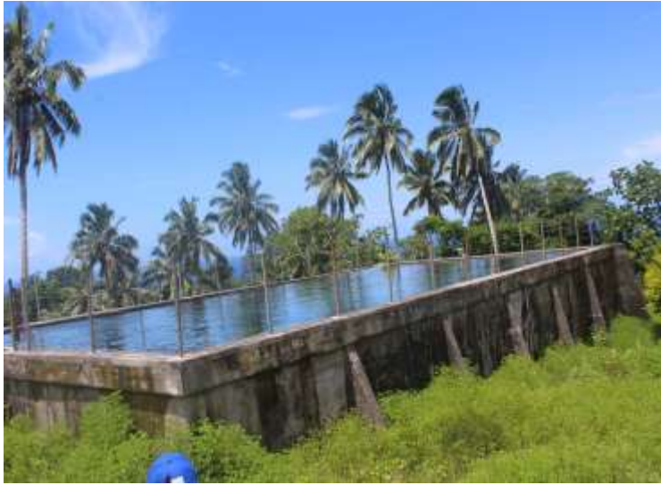
Salailua village water reservoir Independent Water Scheme
