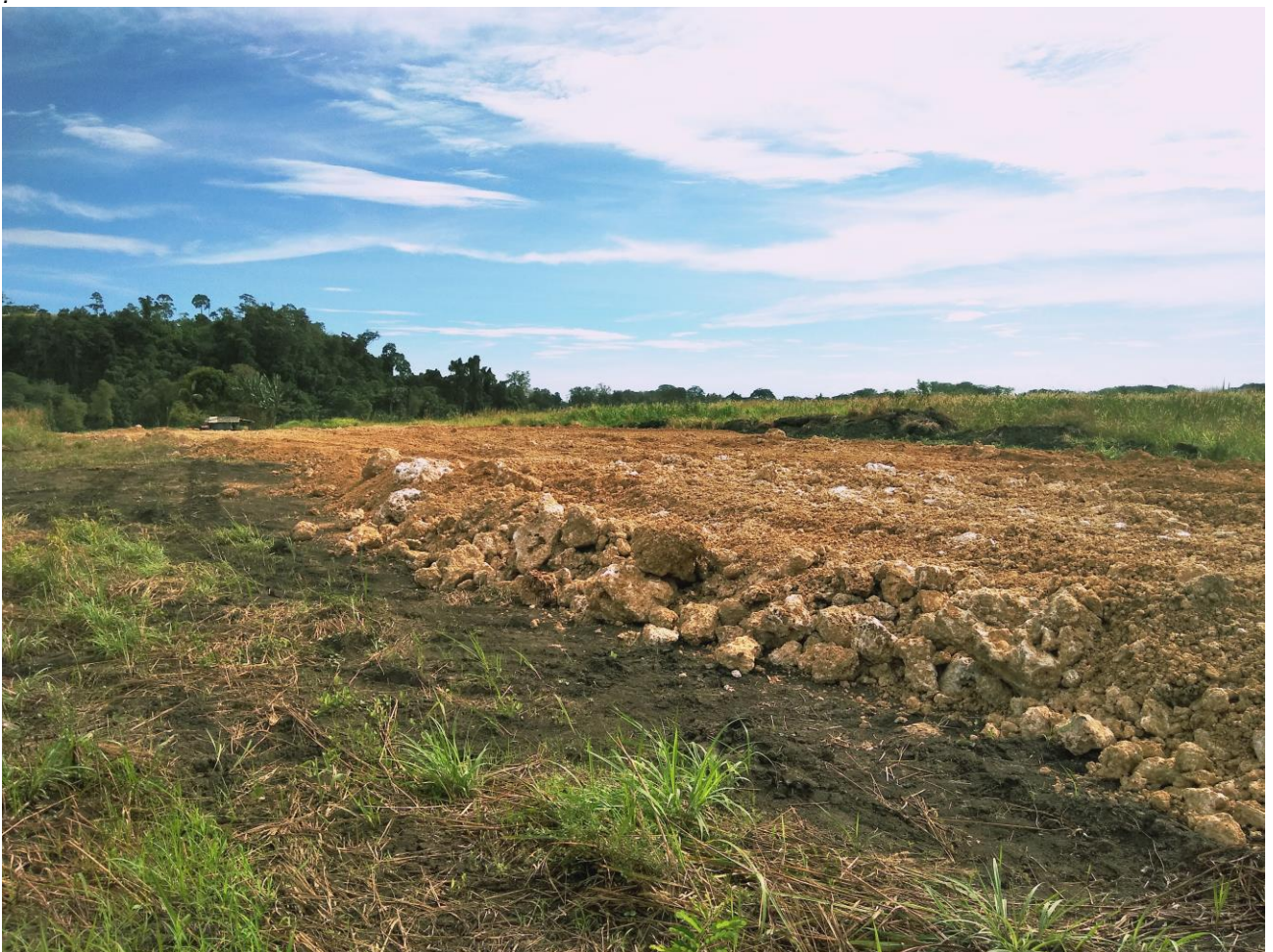
Plate 6. View along formed access, note courageous boulders used to construct road basecourse.
