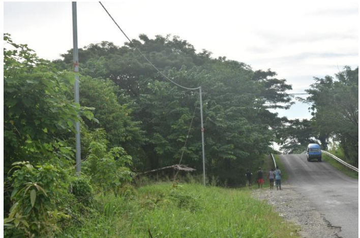
Fig. 21 Power poles ending at Poha
