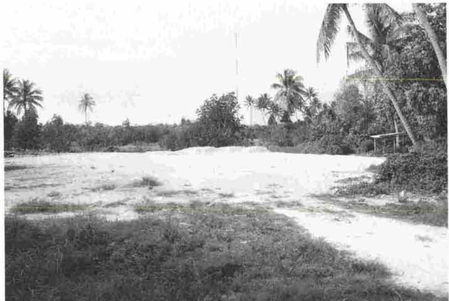
Sand dredged from Funafuti lagoon is used to reclaim low-lying areas. (photo: Alefaio Semese)
