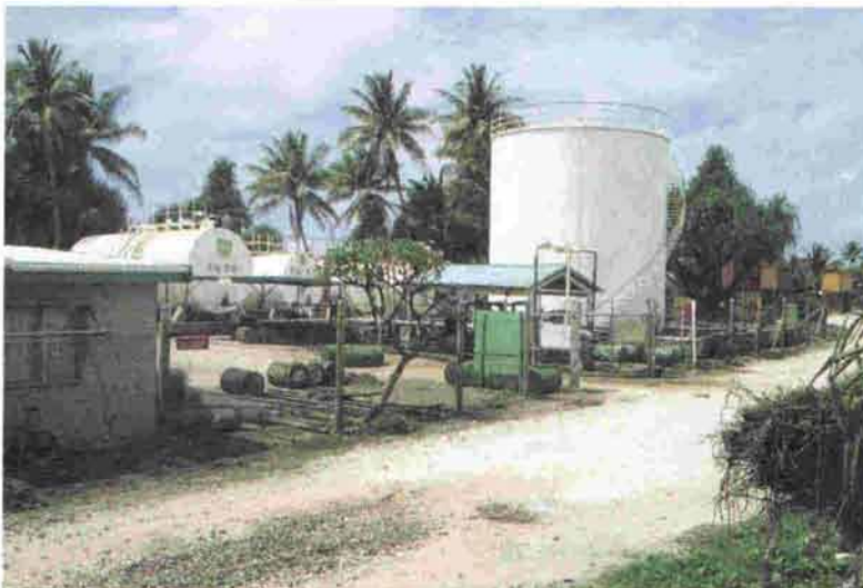
Funafuti BP terminal, where all of Tuvalu's bulk fuel is stored. In this vulnerable environment, it is important to ensure that facilities to cope with oil spills are adequate. (photo: Alefaio Semese)
