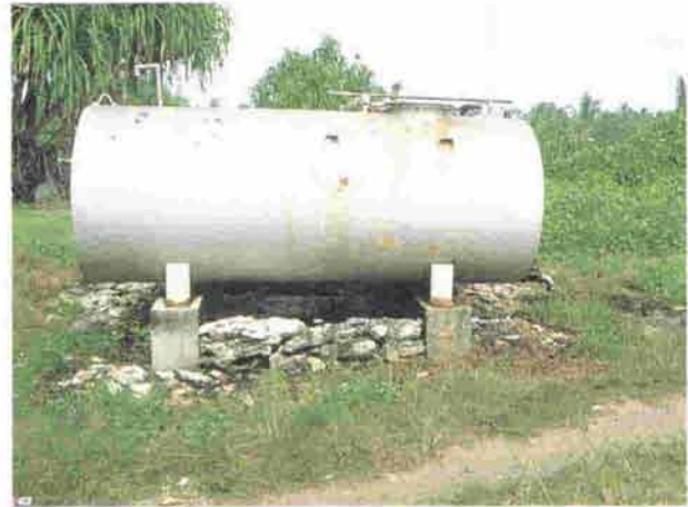
Fuel storage at Funafuti power station. There is no bunding system to retain spillage and no established procedures for cleaning up any spill that might occur. (photo: Alefaio Semese)
