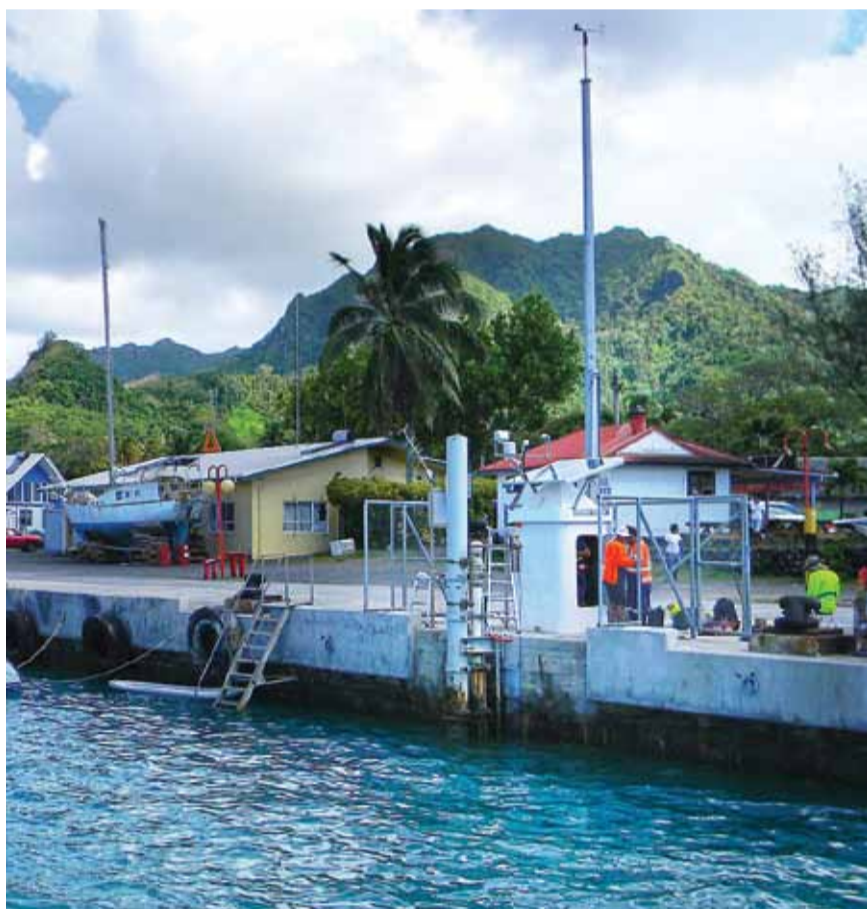
Figure 4. Technicians working on the recently-refurbished Cook Islands tide gauge, which has been monitoring sea level and weather conditions in Rarotonga for over 25 years. Photo: Stamy Criticos (2012).
