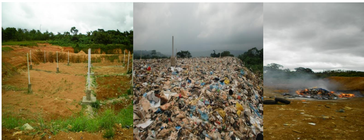
Bouffa semi-aerobic landfill, Port Vila
