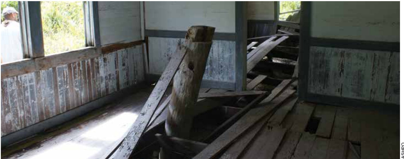
Figure 149: Interior of Jennings house showing wooden pier coming through the floor.
