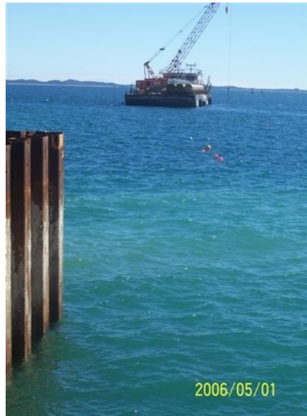
Figure 6: Construction of a sheet pile trench for the Perth seawater desalination plant with minor plume development (by courtesy of Water Corporation of Western Australia).
