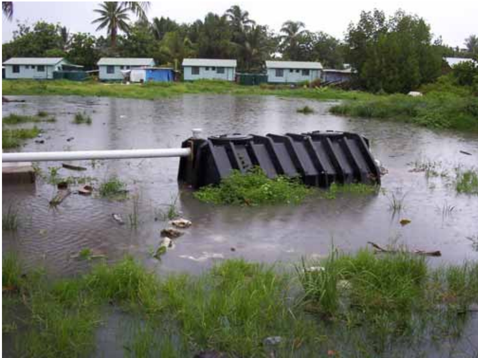
Figure 1a: Regular flooding and poorly designed septic system are major sources of human health and environmental concerns in Tuvalu (Government Housing, Vaifou settlement)
