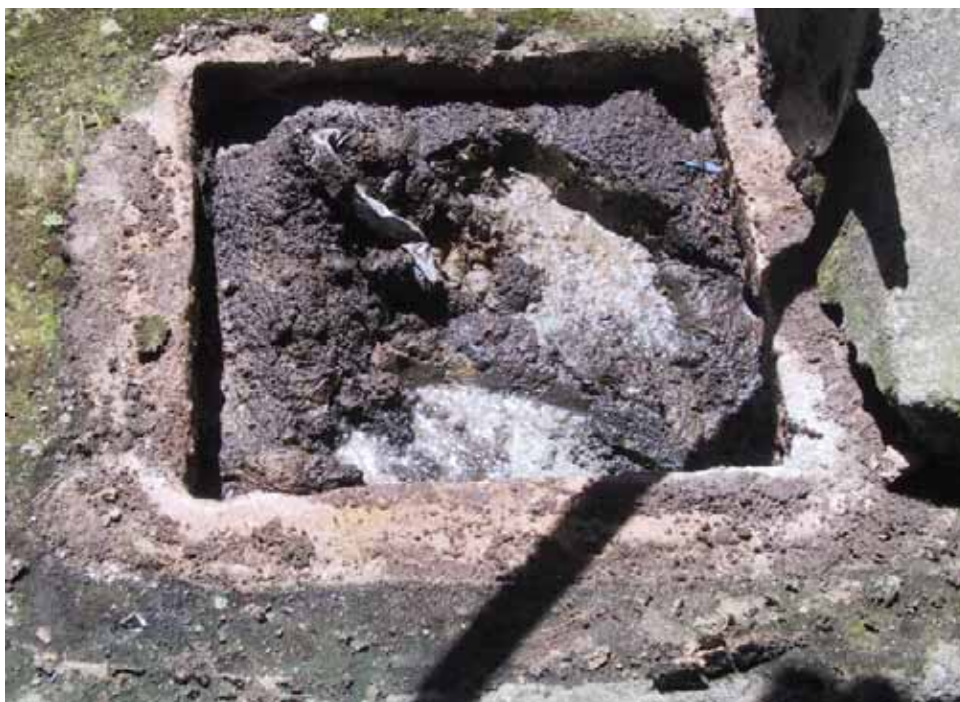
Figure 1D: Poorly maintained tanks (not cleaned until blocked)
