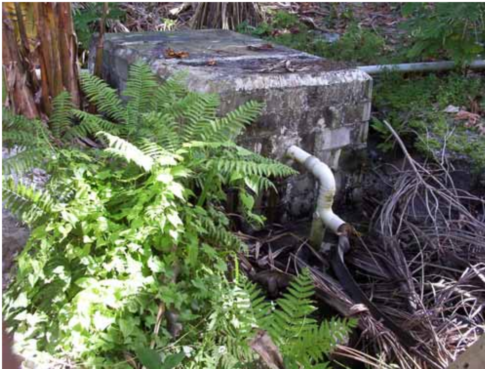
Figure 1C: Poorly designed and installed septic tank
