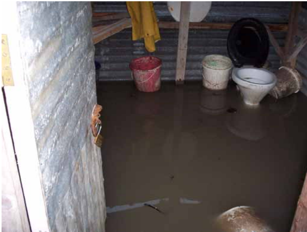
Figure 1B: Flooding inside a house after heavy rains
