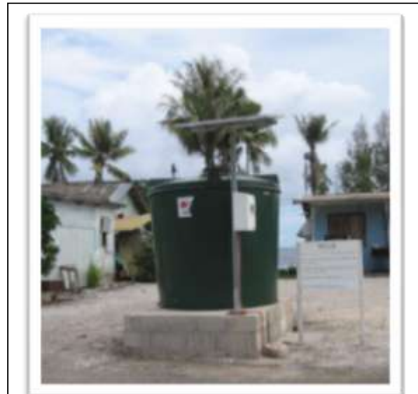
Figure 21: An example of an improved system of water tank with a solar driven water pump. Source: Water Sanitation and Climate Outlook Nauru, SOPAC July 2011.
