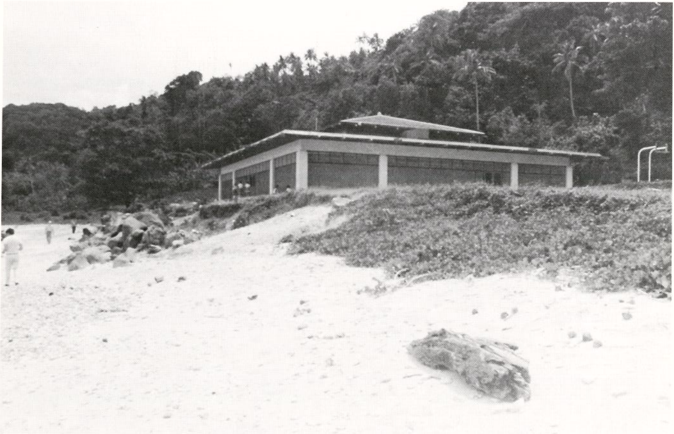
Erosion has washed away the area behind the rock revetment and threatens to undermine the foundation of Poloa School.
