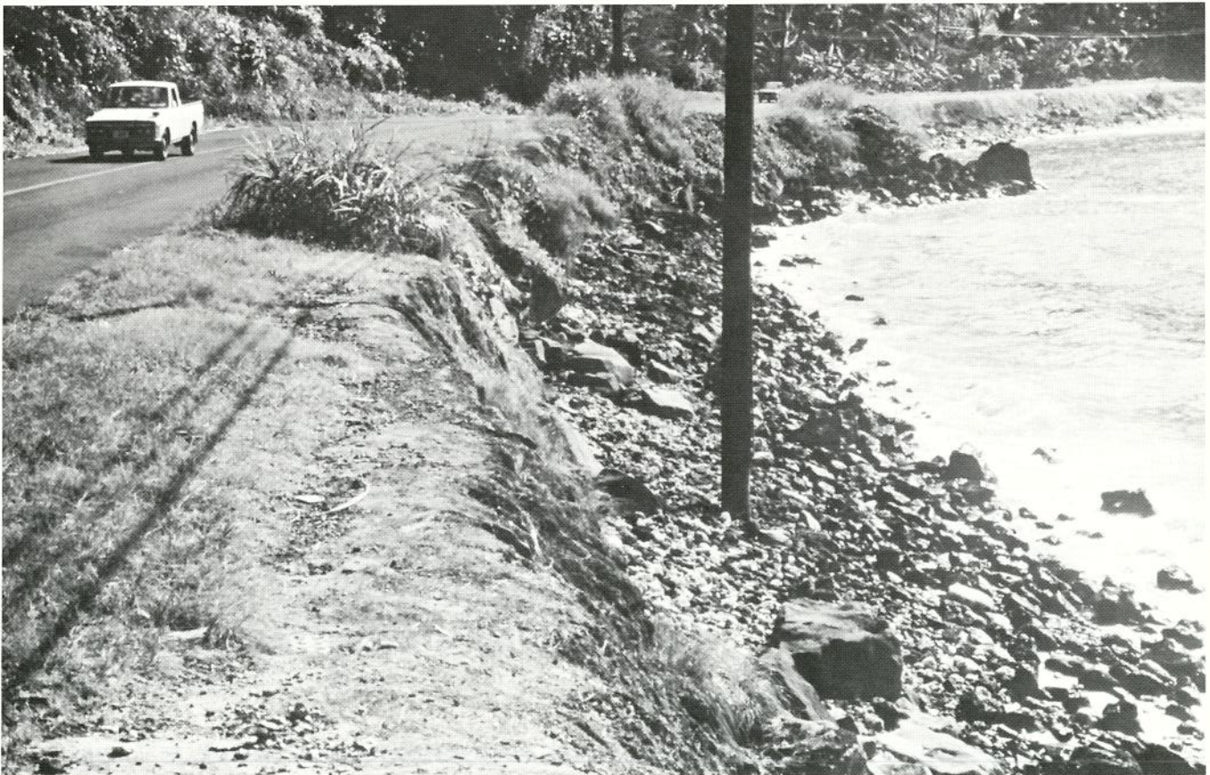
Shoreline erosion between Pago Pago and Nu'uuli threatens utility lines as well as the only highway through this area.
