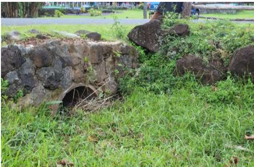
Picture shows the sizing of the pipe culvert across the road is insufficient to accommodate heavy water during flash flood and makes it worse being blocked with weeds and rubbish. (Photo credit: MNRE-PUMA, 2017)
