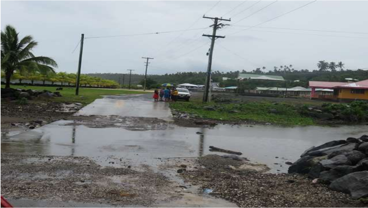
Vaigalu ford crossing Lepa District – community request to replace ford with a bridge
