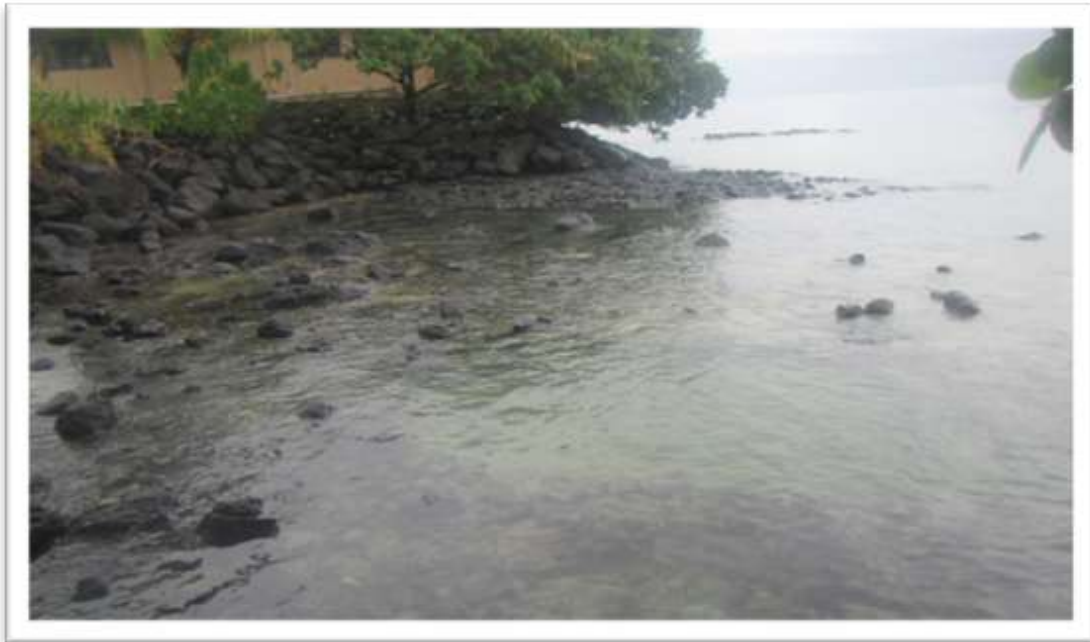
Rock revetment behind residential home on the coast highly eroded due to sea level rise and strong wave action.
