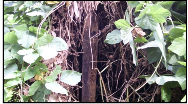
Posts and fence decimated by weeds. Photo Credit: DLVS
