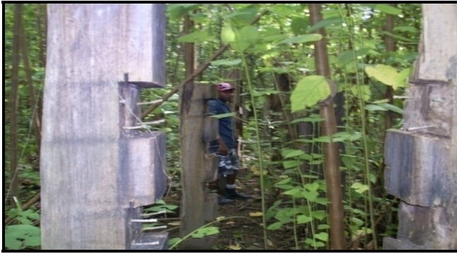
Stockyard with fallen rails, and woody weeds. Photo Credit: DLVS
