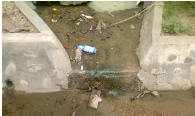
Drains blocked with soil and other waste materials in the Gordens Area Photo © Goije, B., Kioma, T., Bobora, N., Bomai, A. and Kamaso, D. (2012)
