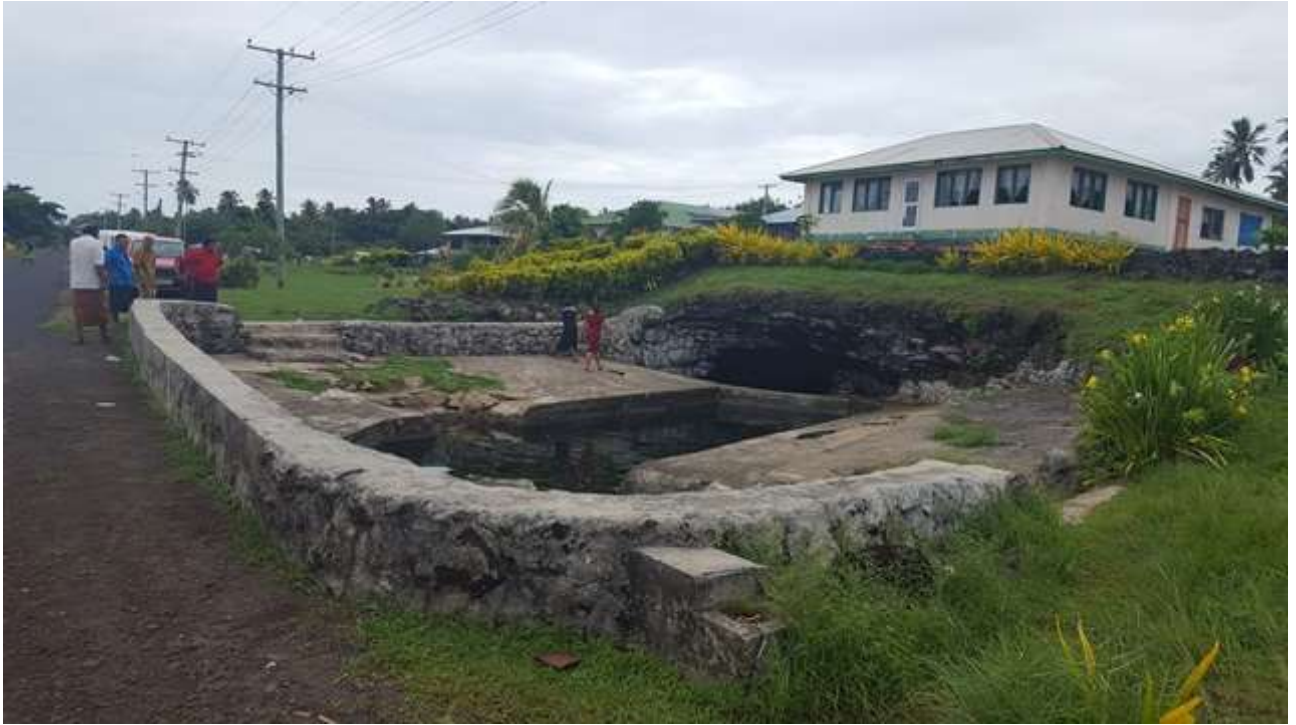
Vailoa coastal spring and drinking water - village request support to repair the wall is deteriorating. Drinking water needs to be tested as there is strong possibility of contamination.
