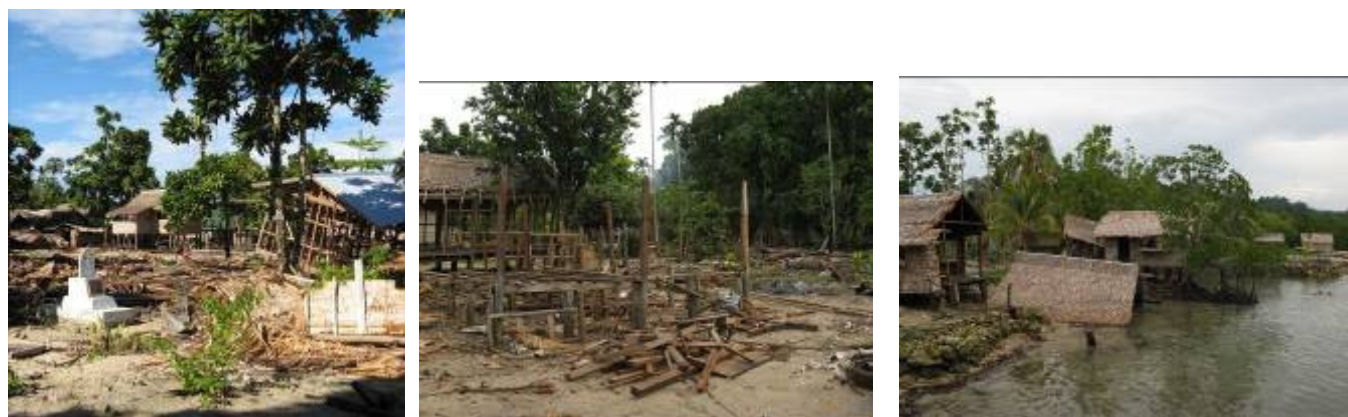
Figure 6. From left to right, damaged homes in Iriqila, Leona and Liangai on Vella Lavella.
