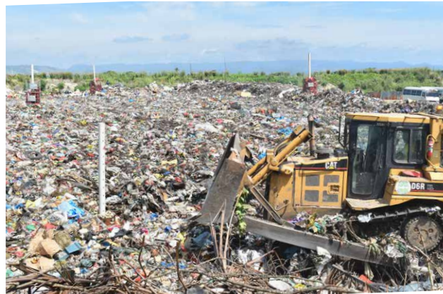
FIGURE 7.1. Bulldozer working at the Ranadi Landfill in Honiara. Gas venting pipes installed at the Landfill made from PVC pipes and locally available materials (© Wendy Beti/ECD 2017).
