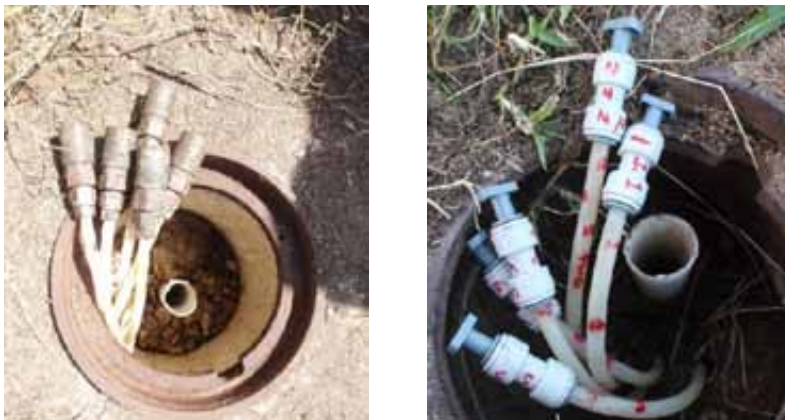
Figure 28: Brass snap couplings (left) were replaced with John Guest fittings (right)
