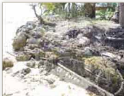
Photo 7: Coastal erosion in Manuka Village, 2006.
