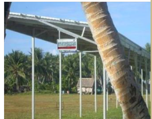
PV solar panels at the secondary school in Vaitupu, peak output 184 W/m 2
