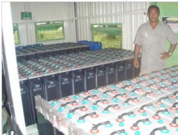
Battery Bank in Vaitupu
