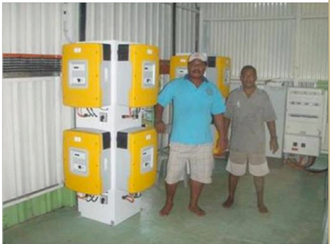
Battery Controls in Vaitupu (SMA)
