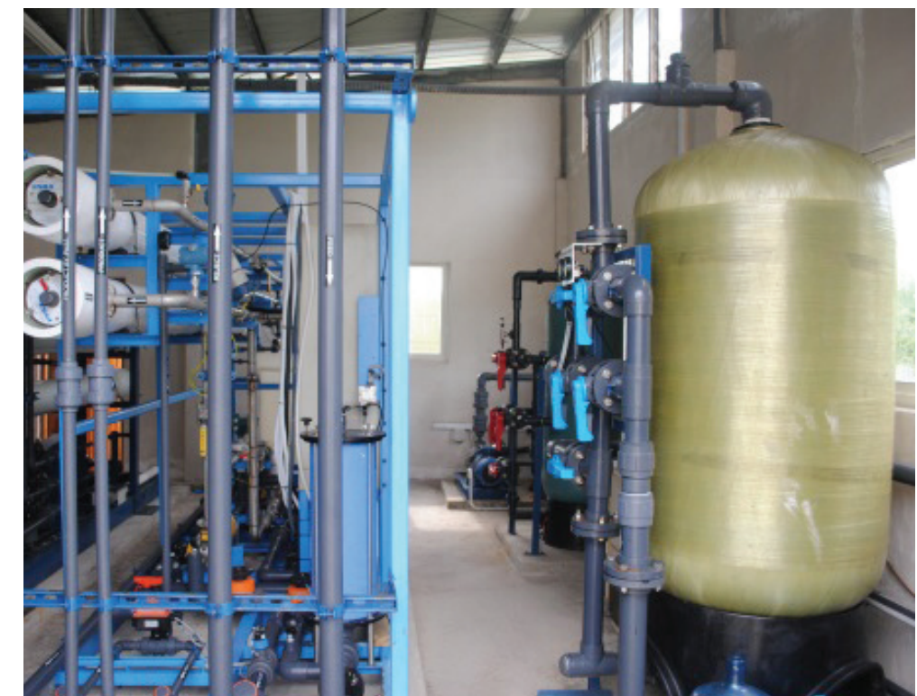
Desalination plant at the Public Works Department depot.
