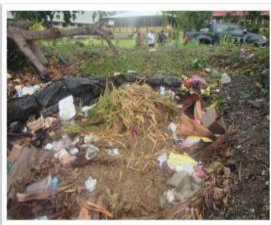
Blocked culvert filled with rubbish dumped across the road limiting the flow of storm water into the sea and causing flooding - Faleasiu
