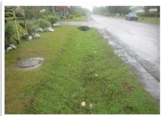
Shallow drainage system and narrow culverts along the main road (West Coast Road) at Faleasiu (sub-village Sapulu) during rainy season it overflows and flood and most coastal residential area
