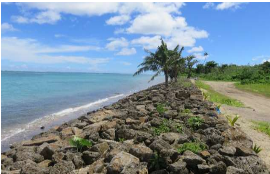
Seawall recently completed in Malaemalu has shown very weak and poor loose structure, strong potential to have adverse impact on marine environment.
