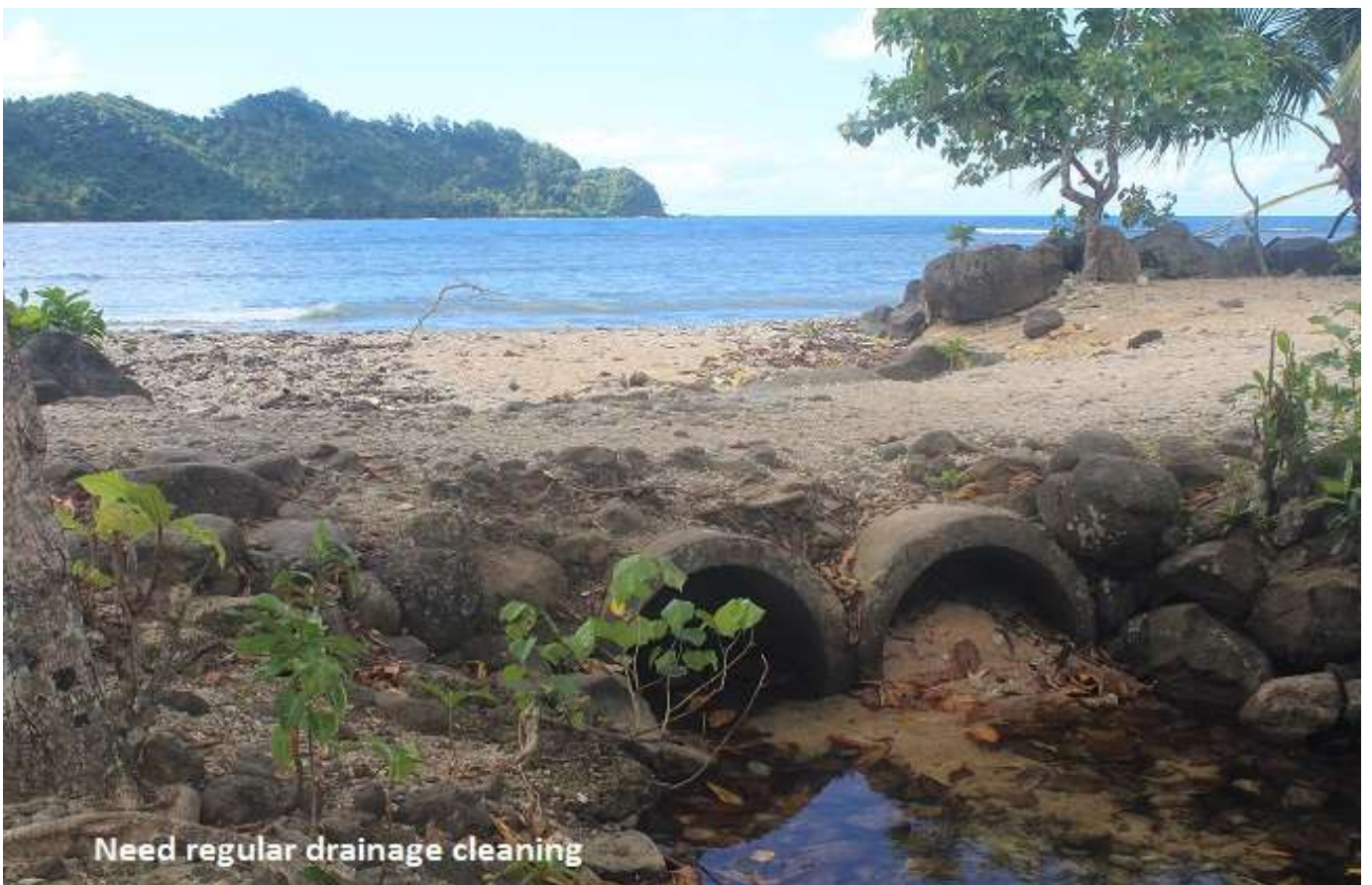
Maintain or upgrade ford to a bridge to improve accessibility during natural hazards
